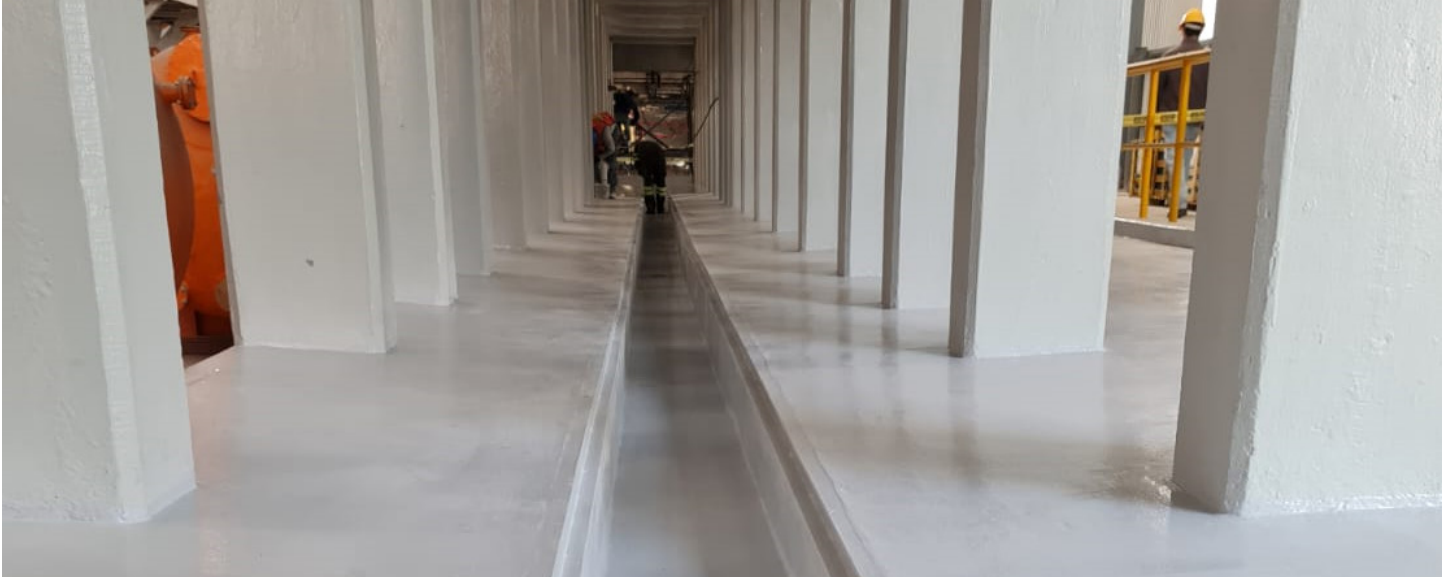
2. Floor, Wall, and Column Coating Installation – A lighter-duty, fiberglass reinforced coating on the columns and floor underneath the elevated pickling line platform.
